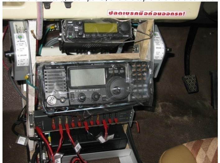
Radio Console (top to bottom/left to right): HF antenna switch, VHF radio, VHF antenna switch; HF radio, 12 VDC power distribution panel, antenna tuner.
