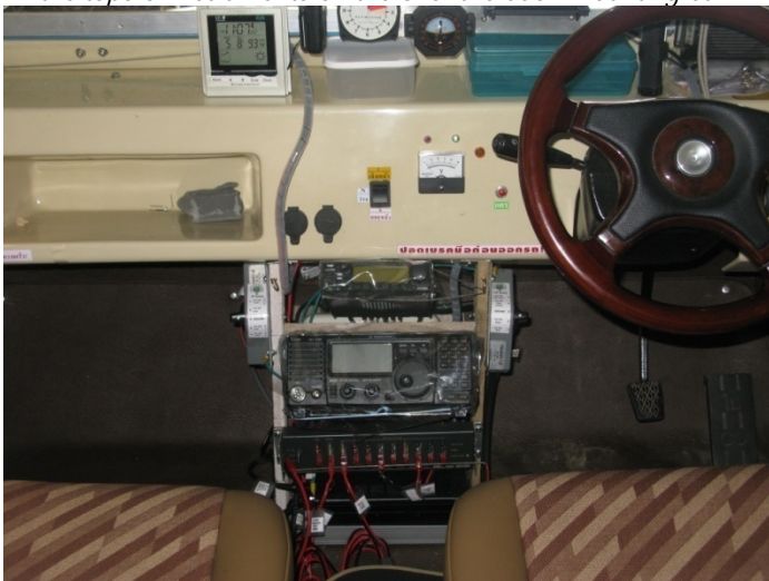
The radio console contains the radios, antenna switches, 12 VDC power panel and antenna tuners. Station ground bus panel is on the interior firewall directly behind the radio console.
