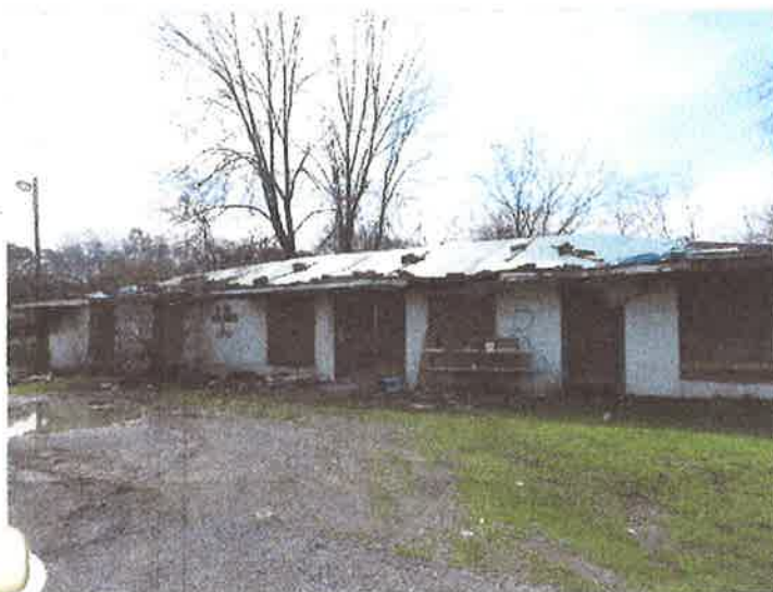
This crumbling old store covered with tarps sits...
