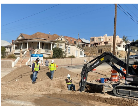
The Upson Drive Main Improvement Project in Sunset Heights will reduce breakages and disruptions.
